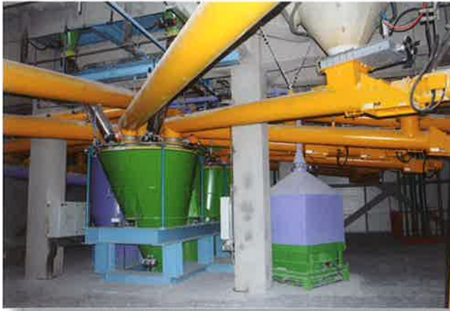
Figure 3. Main material hopper scale with dosing screw conveyors
