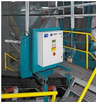
EIRICH QualiMaster AT1 for testing of the molding sand quality
