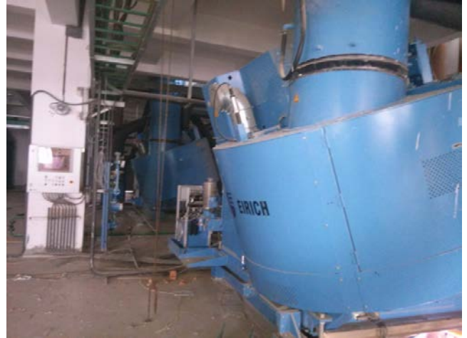
Fig 9: Remixer-cooler 2 x 35 t/h
